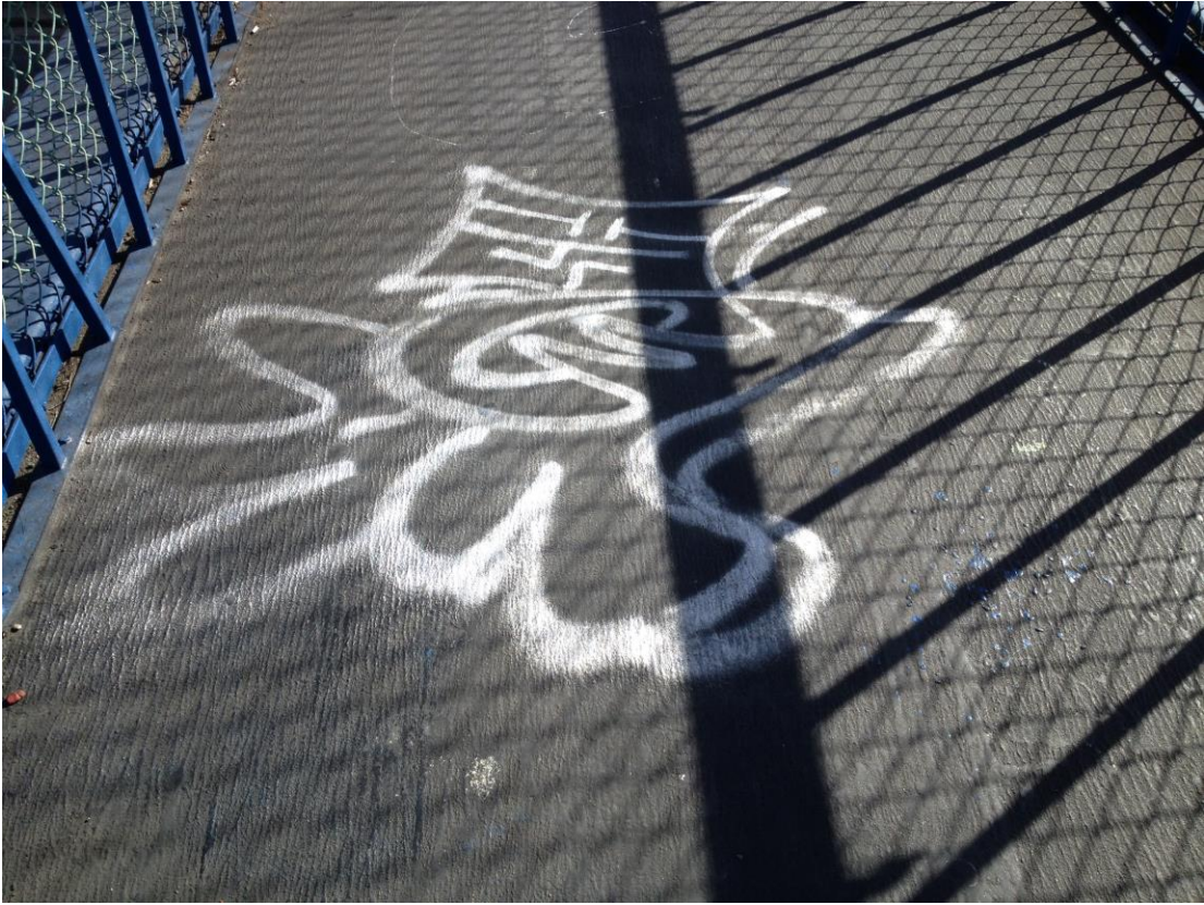
Floor of 18 th Street Pedestrian Overpass – 18 th between Utah and San Bruno
