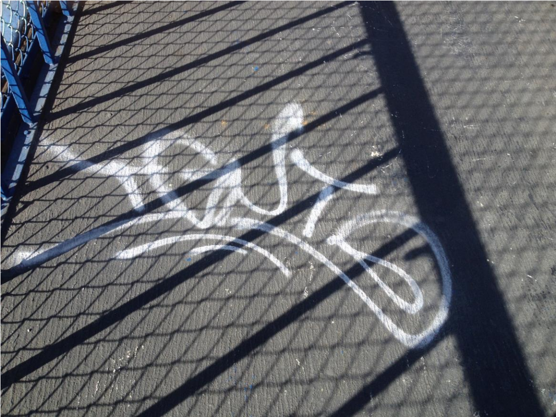
Floor of 18 th Street Pedestrian Overpass – 18 th between Utah and San Bruno
