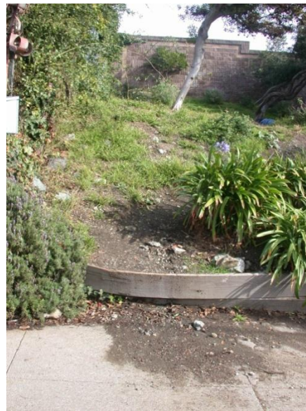
Broken retaining wall built in 1970
